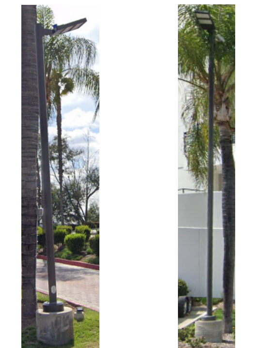
Existing Pole Top - 18' Existing Pole Top - 30'
