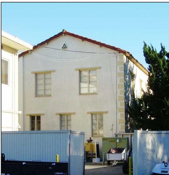
Part of the north elevation (1/21/11). Part of the Fire Station building is in the foreground (left side of the photograph).
