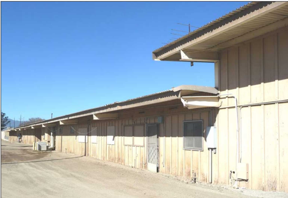
View to the northeast, note the boarded up windows (1/21/11).
