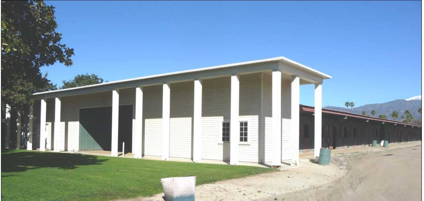
Southwest end of HRS #1 (closest to the race track), view to the north showing later alteration (1/21/2011)
