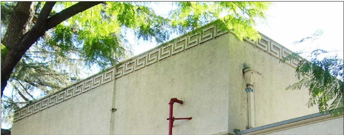
Figure 23: Millard Sheets Building detail; decorative pattern along the top of the building wall, eastern elevation near the southern end of the building (1/21/11).
