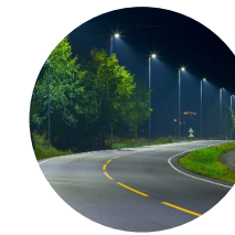
Upgrade Street Lighting (install new street light poles) Enhance Nighttime Visibility & Safety
