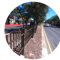
Install Median with Curb & Gutter Reduce Left Turn Conflicts & Enhance Roadway Safety
