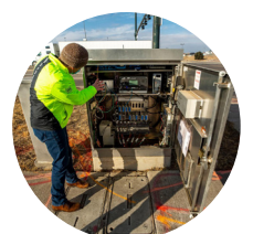
New Signal Hardware Enhance Signal Visibility, Operations & Safety
