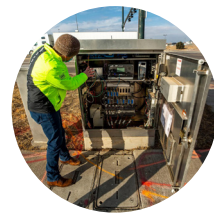
New Signal Hardware Enhance Signal Visibility, Operations & Safety
