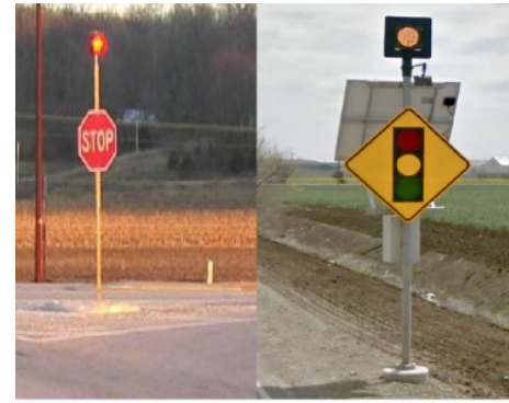
INSTALL FLASHING BEACONS AS ADVANCE WARNING
