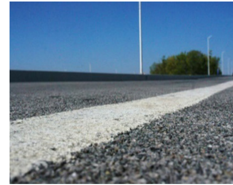
IMPROVE PAVEMENT FRICTION (HIGH FRICTION SURFACE TREATMENTS)
